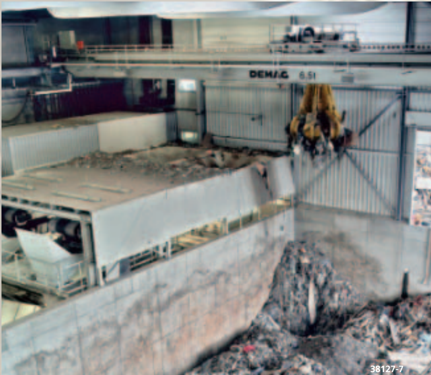
When the going gets tough Double-girder open-winch crane with refuse grab in a pelletising plant.
